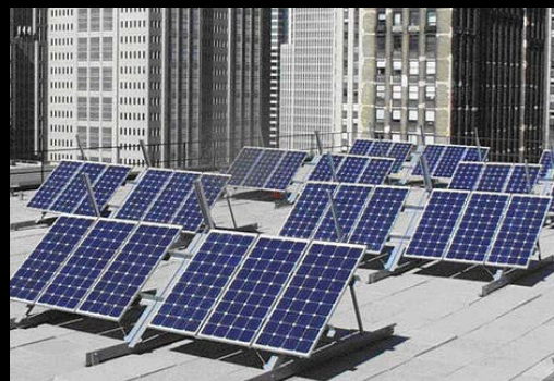
~5 kW roof top system
